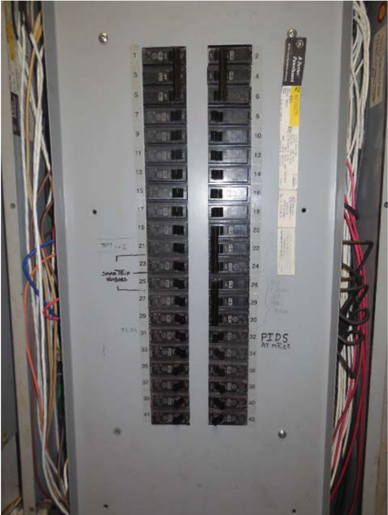
Picture 3: F08 Southern Ave - Panel MESS in Room C205
