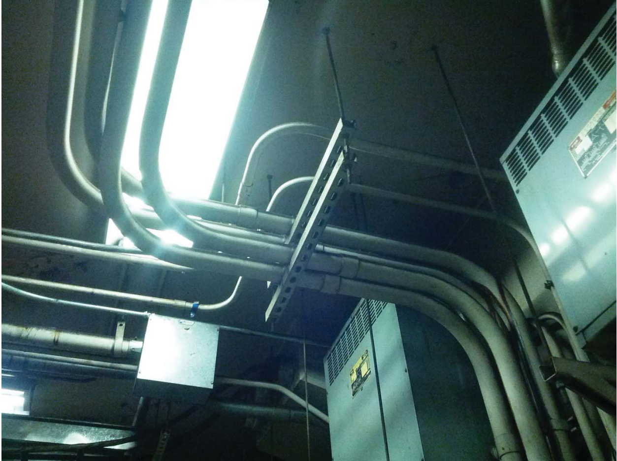
L'Enfant Plaza North Photo #6 –AFC Panel (NF) – Overhead Conduit Transition (Platform Level Rm. N104)
