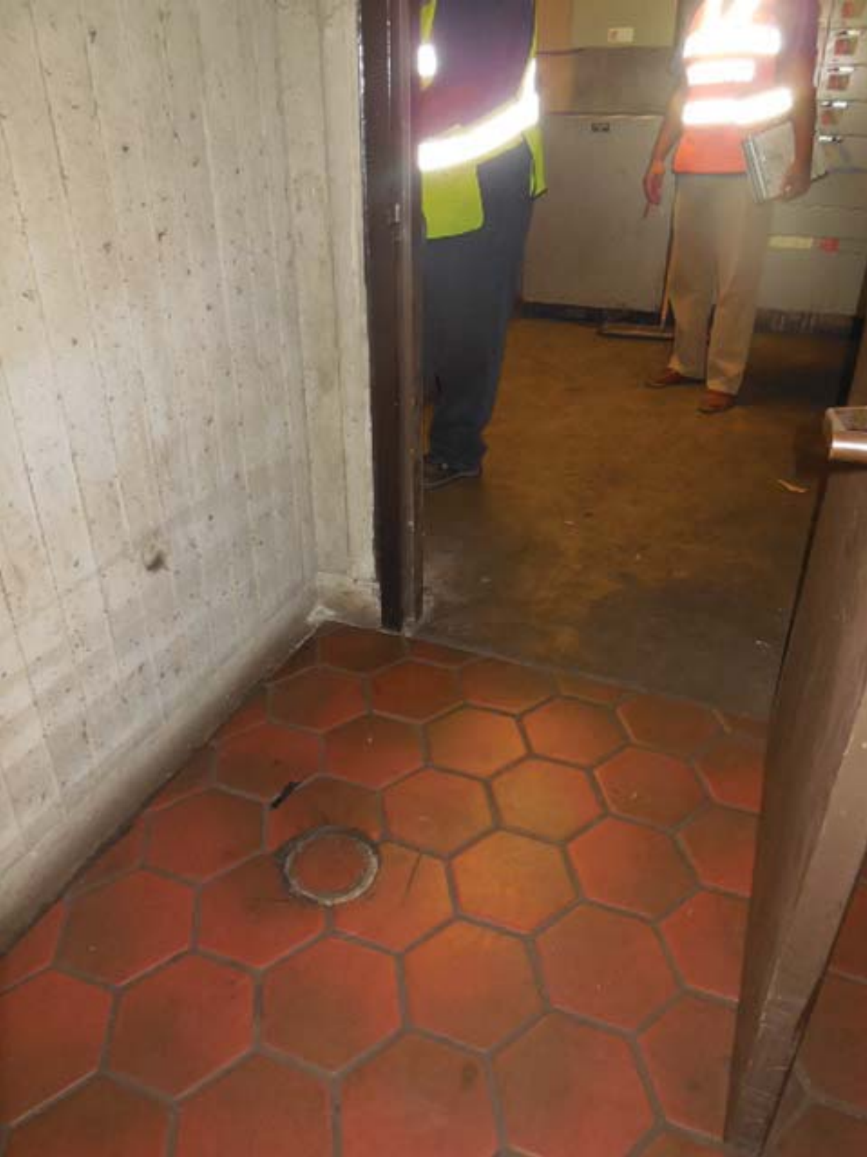
Picture 3: F07 Congress Heights – Handholes near door to Rm C216 from Mezzanine
