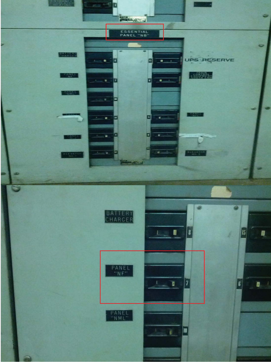
L'Enfant Plaza North Photo #10 – AFC Source Switchboard (NB) located in Room #N104 on Platform Level Track 2 Wayside. Source Breaker (Panel “NF”) Circuit #7 for AFC Panel (NF).
