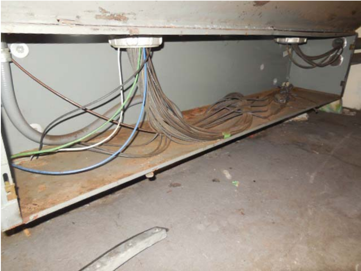
Picture 13: F04 Waterfront – Panel MESS-1 shared trough in Room C206
