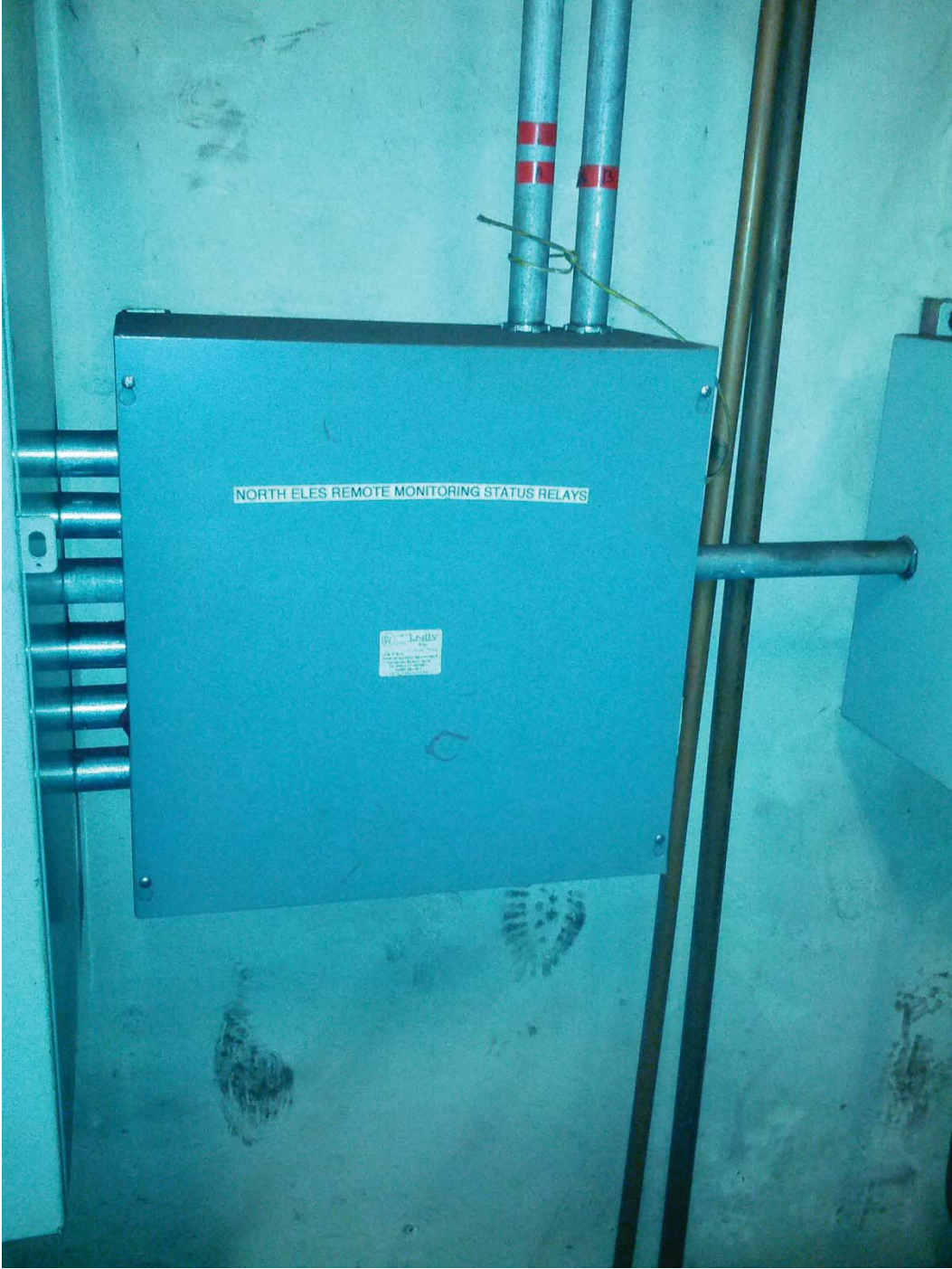
L'Enfant Plaza North Photo #11 – North ELES Remote Monitoring Status Relays – Panel Shares Junction Box (shared raceway) with AFC Panel (NF).
