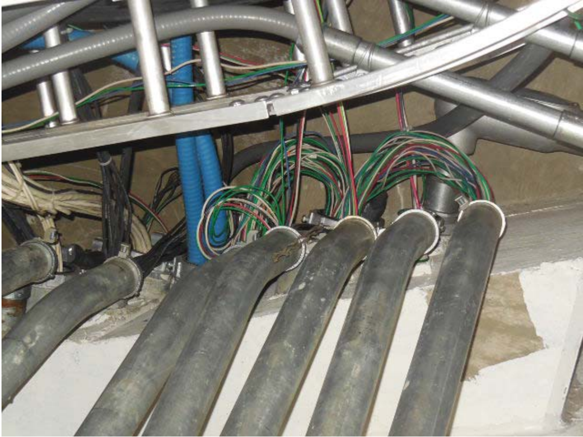
Photo #3: F05 Navy Yard (West) – Conduit transition near the ceiling from panel WMESS in Room 401
