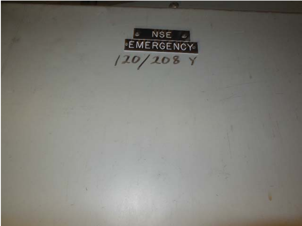
Pictures 8&9: F06 Anacostia (North) – Emergency Panel NSE in room 301
