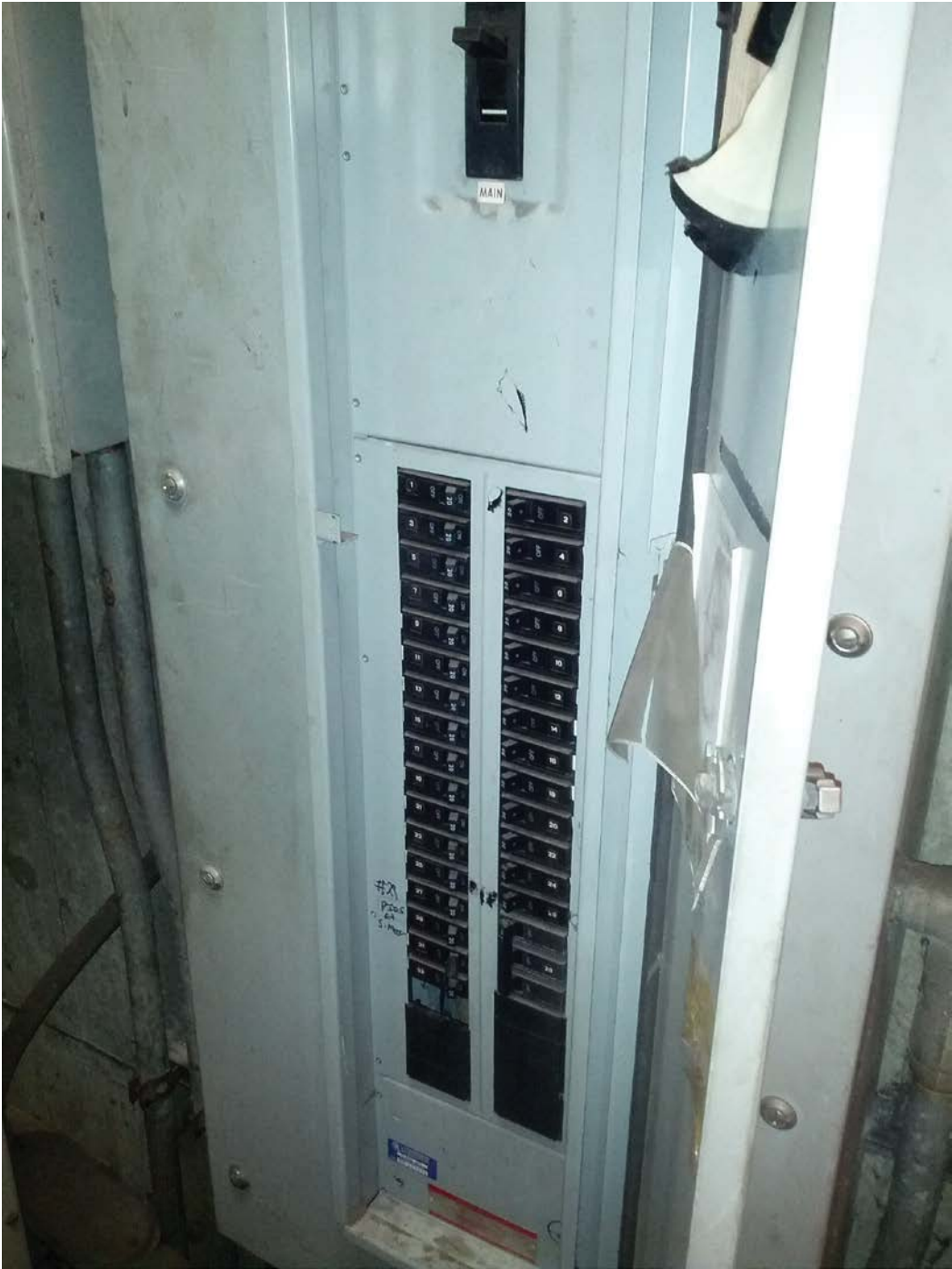
Picture 5: F06 Anacostia (South) – AFC Panel SSF in room 302
