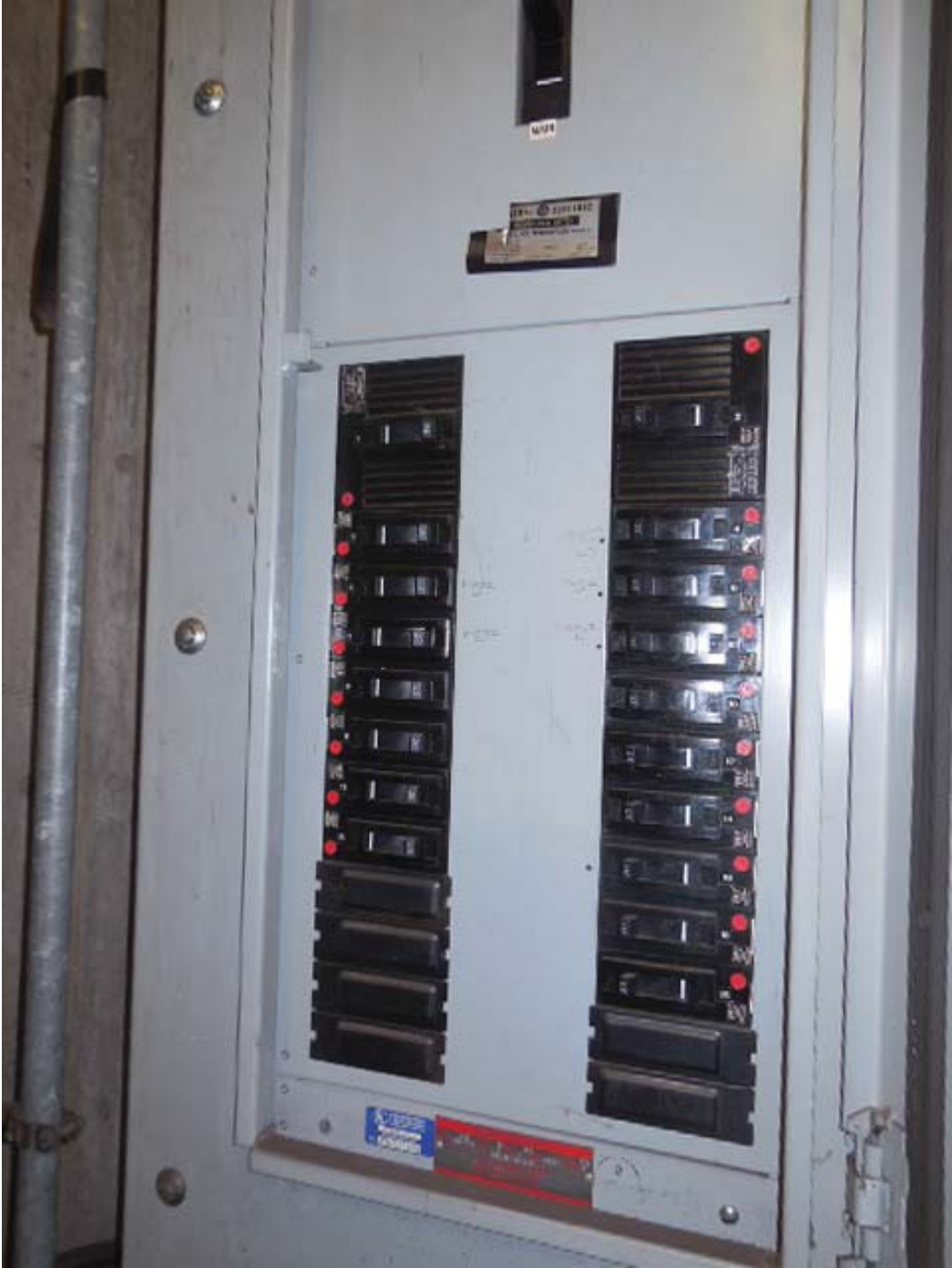
Picture 9: F06 Anacostia (South) – Panel SSM in room 302
