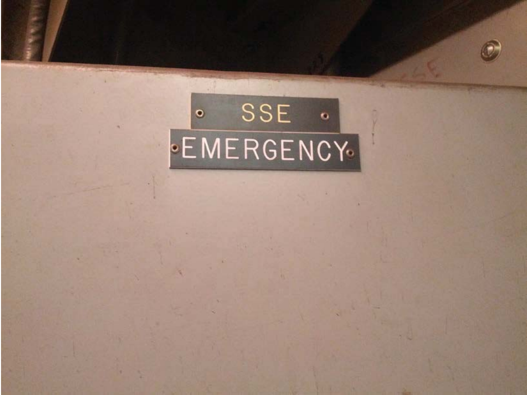
Picture 11: F06 Anacostia (South) – Panel SSE Emergency in room 302
