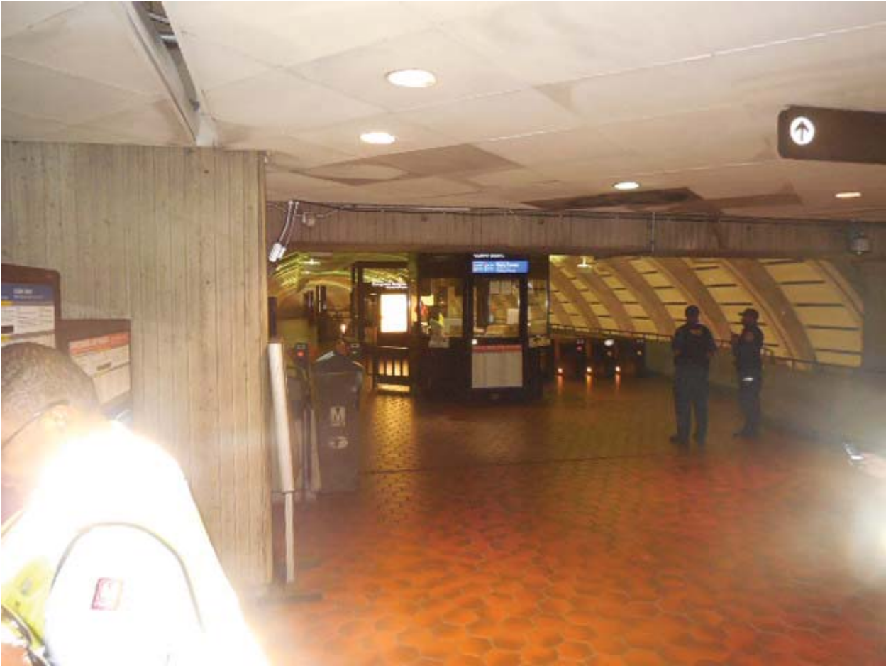
Picture 2: F07 Congress Heights – Handholes believed to be under fare vending machines in Mezzanine
