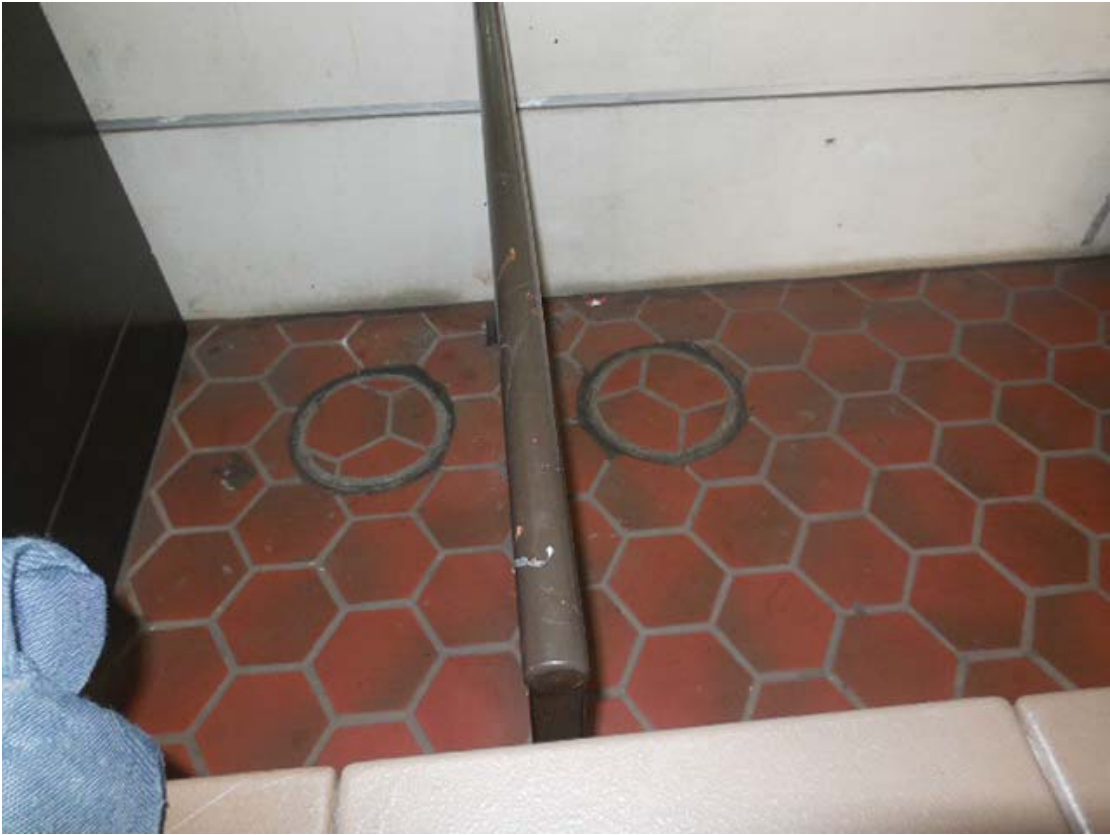
Photo #2: F05 Navy Yard (West) – Handholes at mezzanine level
