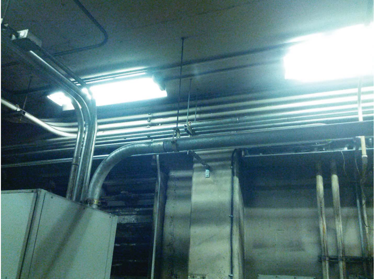
L'Enfant Plaza North Photo #8 –AFC Panel (NF) – Overhead Conduit Transition (Platform Level Rm. N104)
