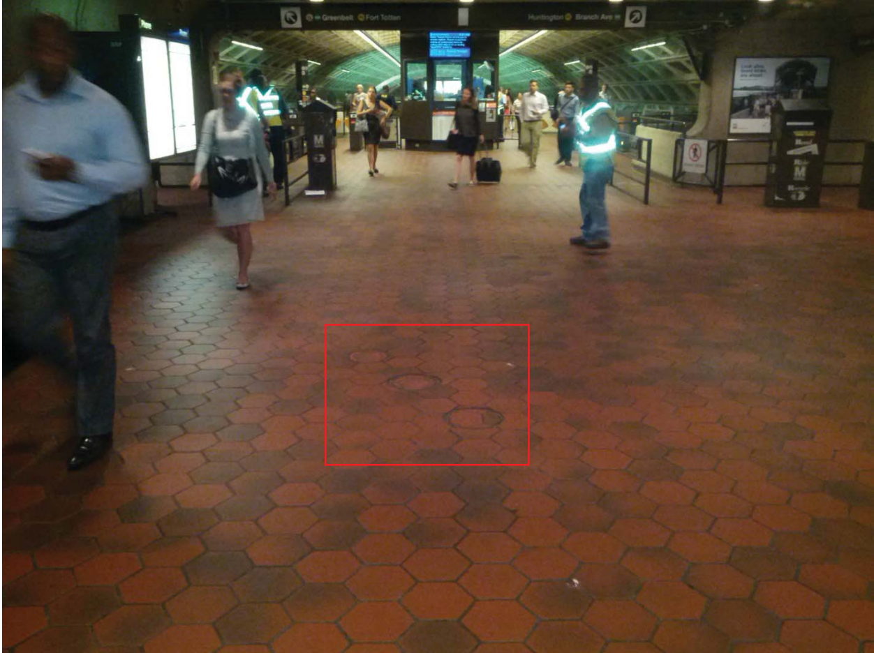
L'Enfant Plaza North Photo #16 – Handholes located on Mezzanine level about 60' feet from Kiosk
