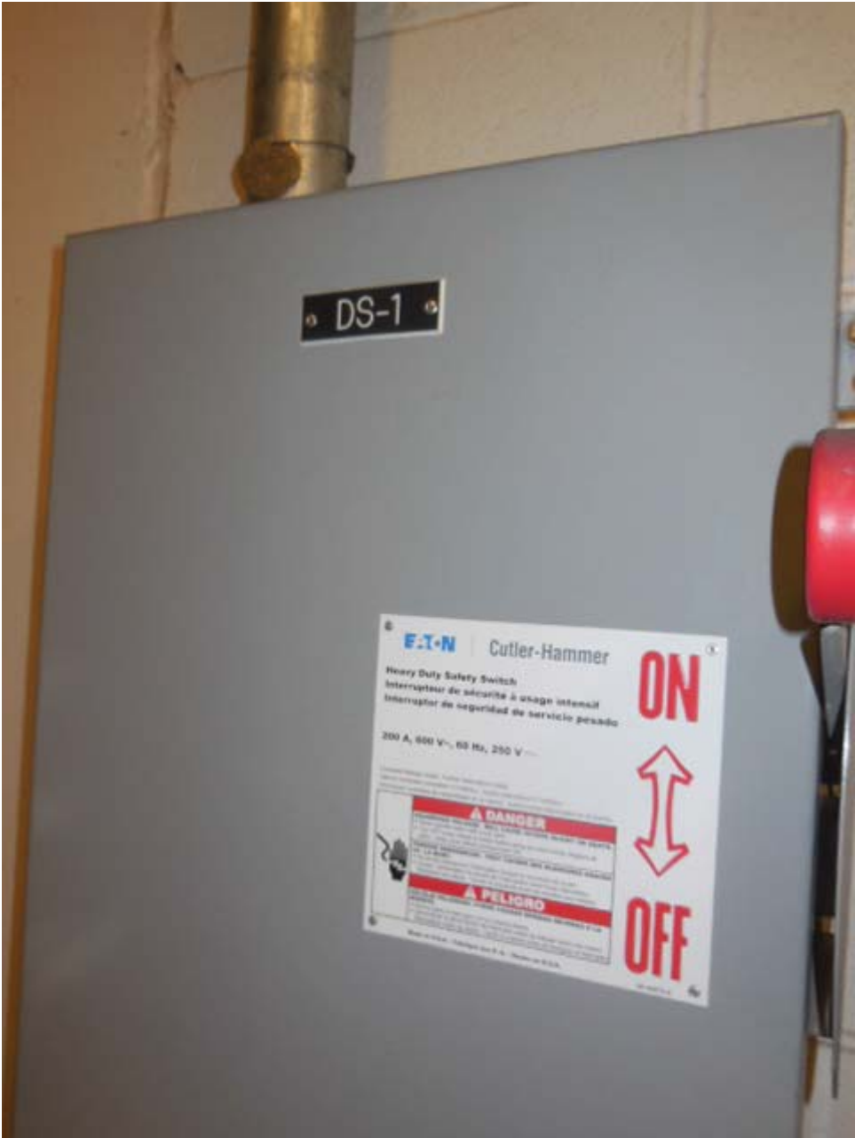
Photo #1: F05 Navy Yard (West) – Panel Disconnect Switch DS-1
