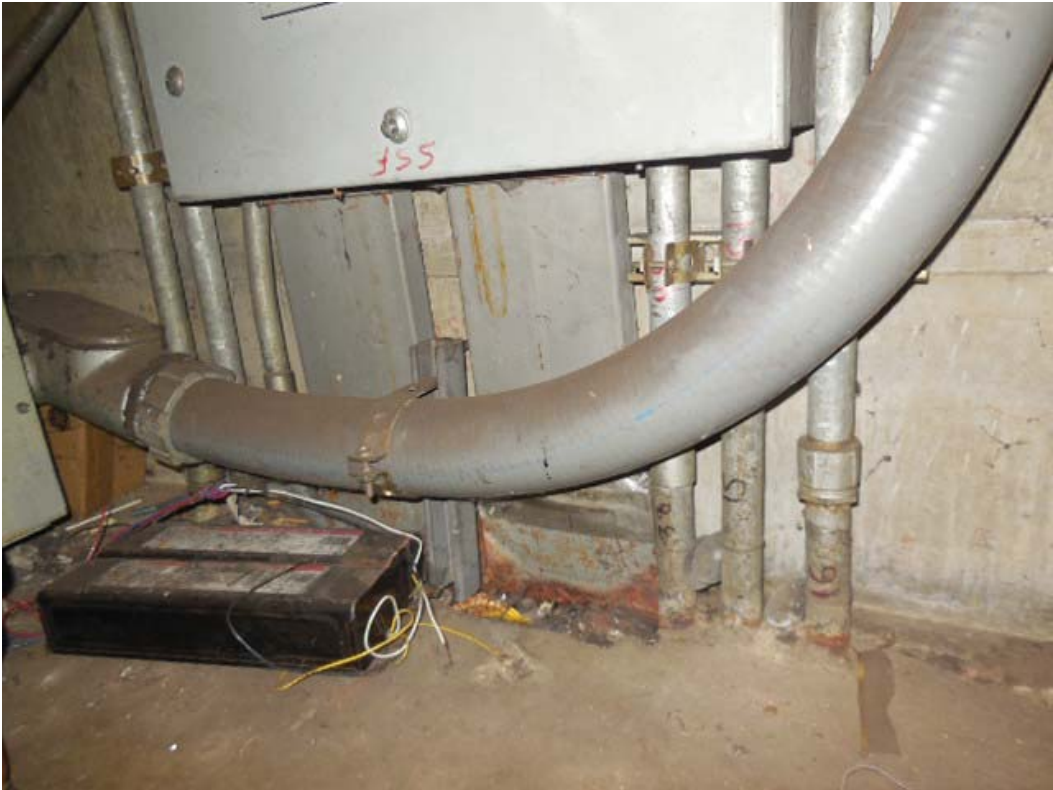
Picture 6: F06 Anacostia (South) – AFC Panel SSF in room 302, bottom ducts
