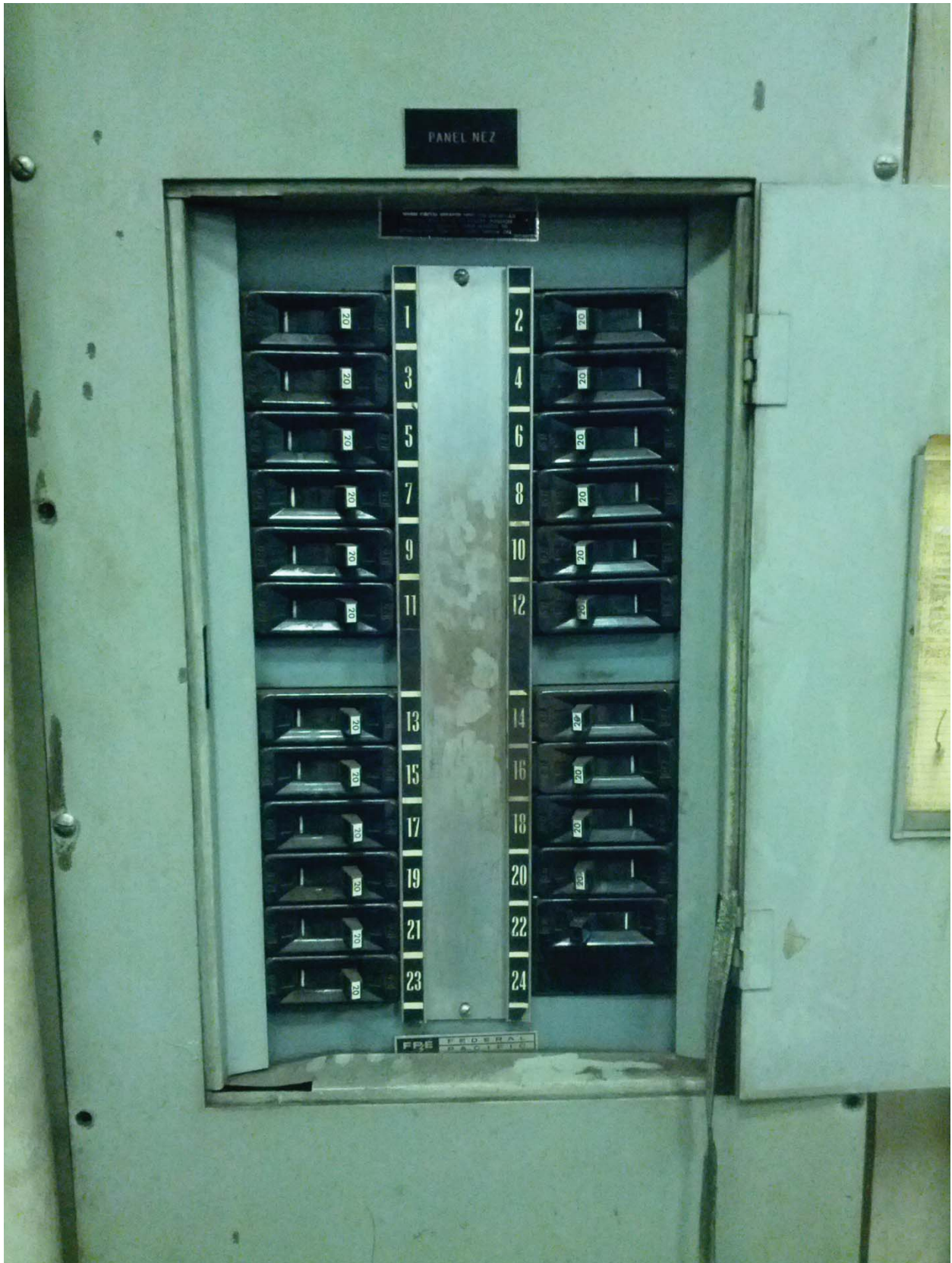
L'Enfant Plaza North Photo #12 – Panel NEZ Serves North ELES Remote Monitoring Status Relays Panel
