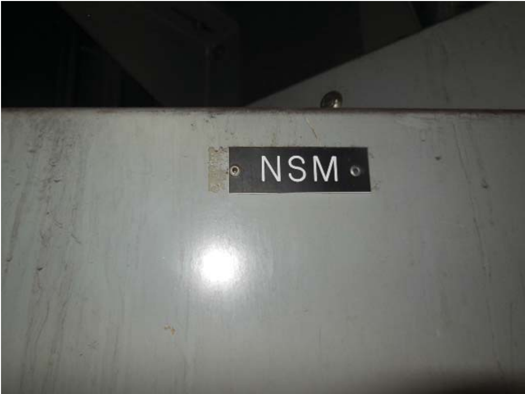
Picture 6: F06 Anacostia (North) – Panel NSM in room 301
