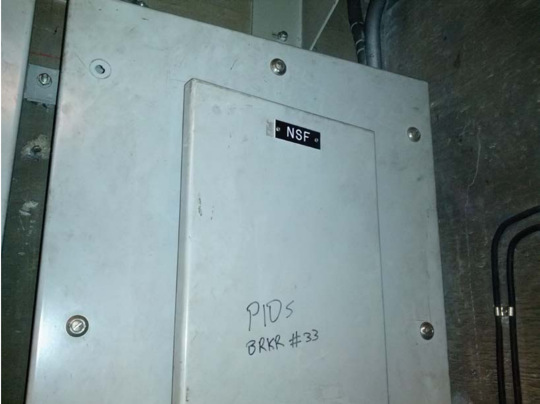
Picture 2: F06 Anacostia (North) – AFC Panel NSF in room 301
