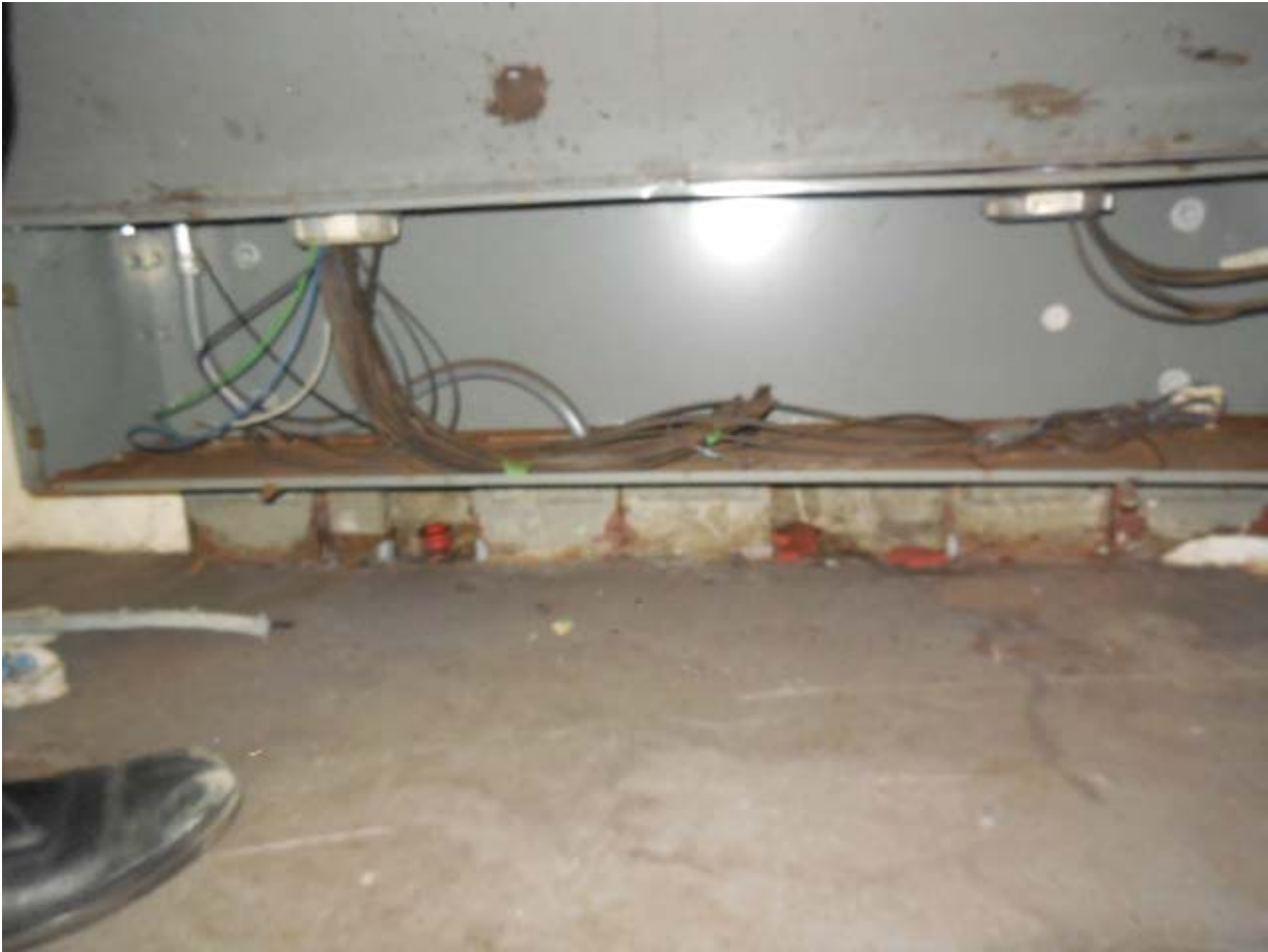
Picture 12: F04 Waterfront – Panel MESS-1 shared trough in Room C206
