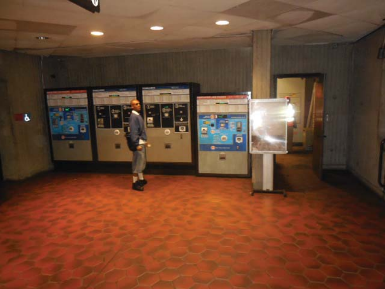
Picture 1: F07 Congress Heights – Handholes believed to be under fare vending machines in Mezzanine
