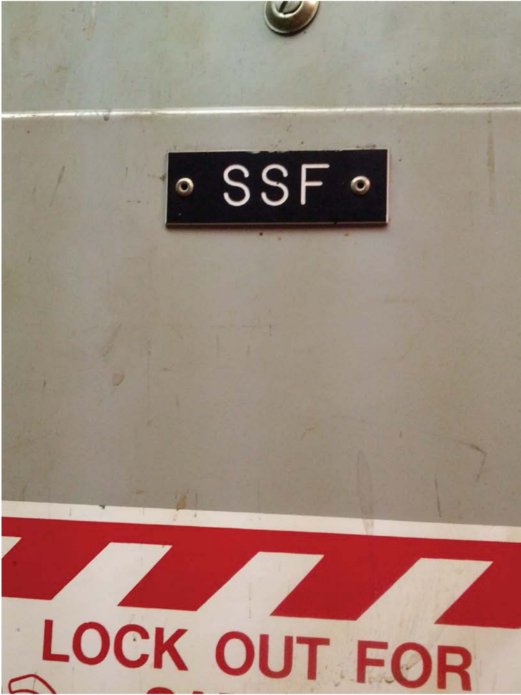
Picture 4: F06 Anacostia (South) – AFC Panel SSF in room 302
