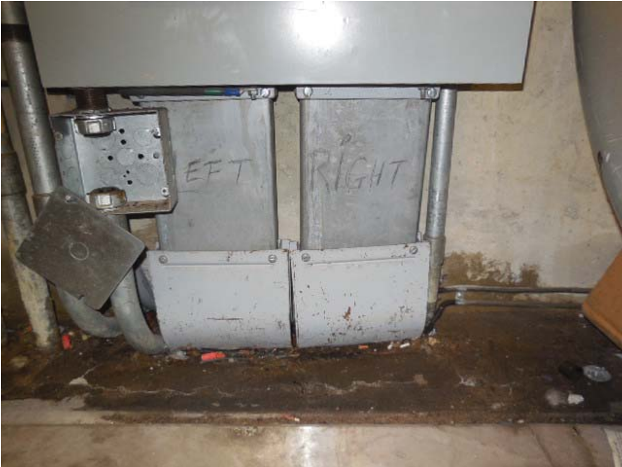
Picture 4: F08 Southern Ave – Bottom ducts of Panel MESS in Room C205
