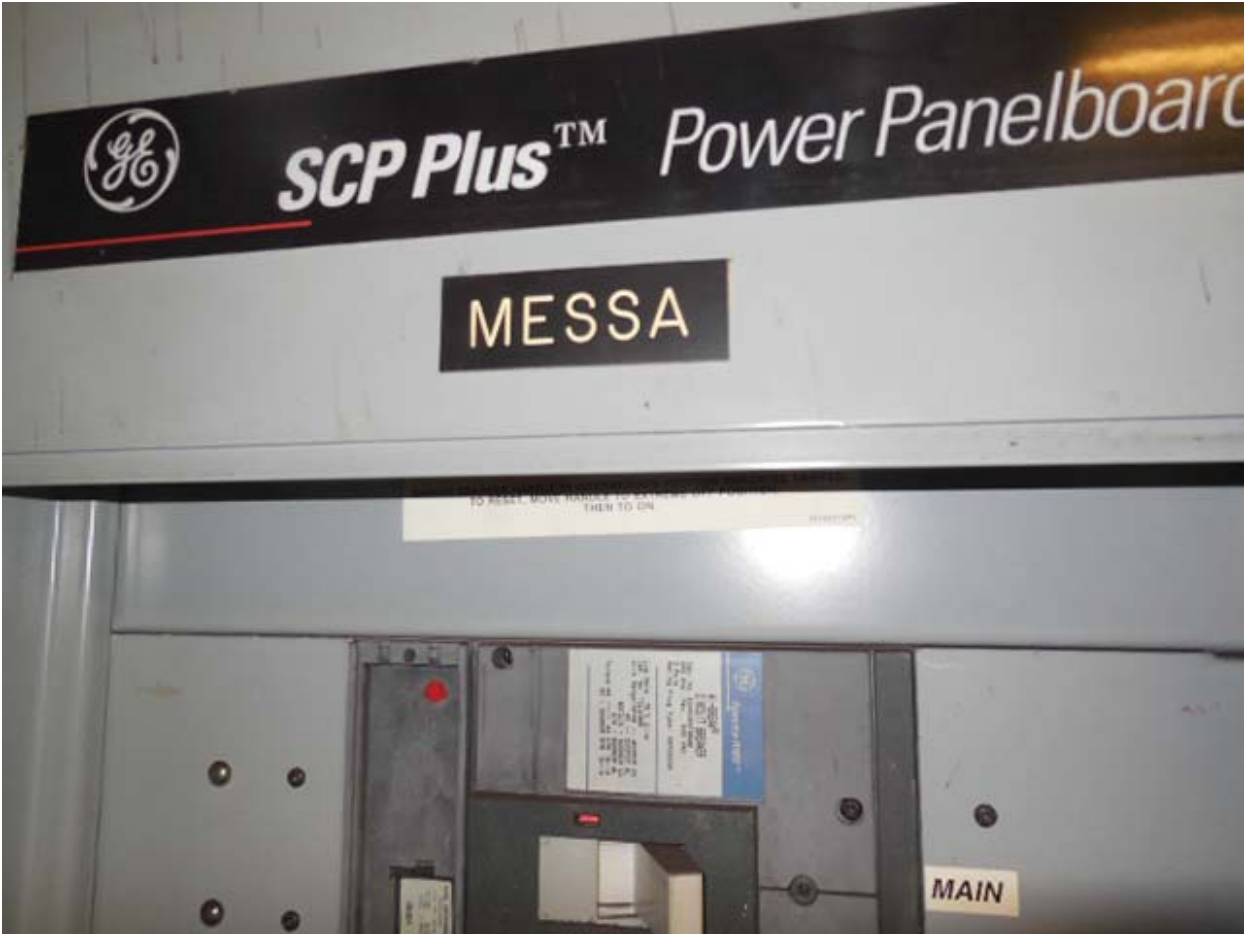
Picture 8: F07 Congress Heights – Source Panel MESSA in Room C216
