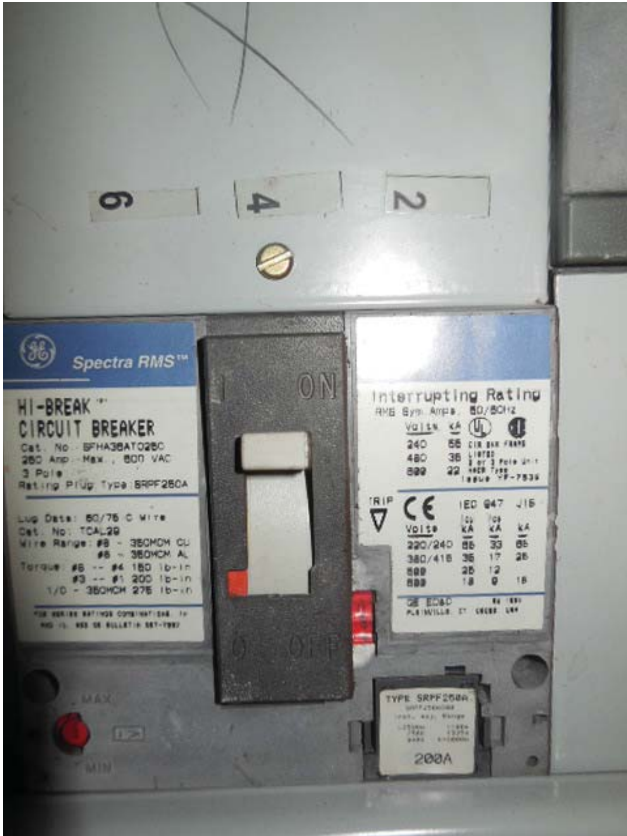
Picture 9: F07 Congress Heights – Source Panel MESSA circuits 2,4,6 in Room C216
