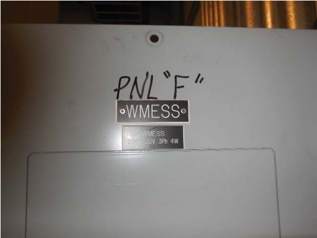
Photo #5: F05 Navy Yard (West) – Panel WMESS Label in Room 401
