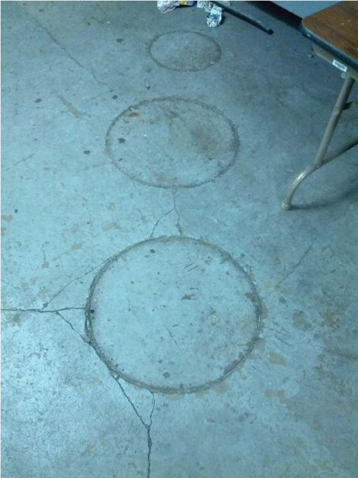
Picture 5: F04 Waterfront – Room C206 manholes
