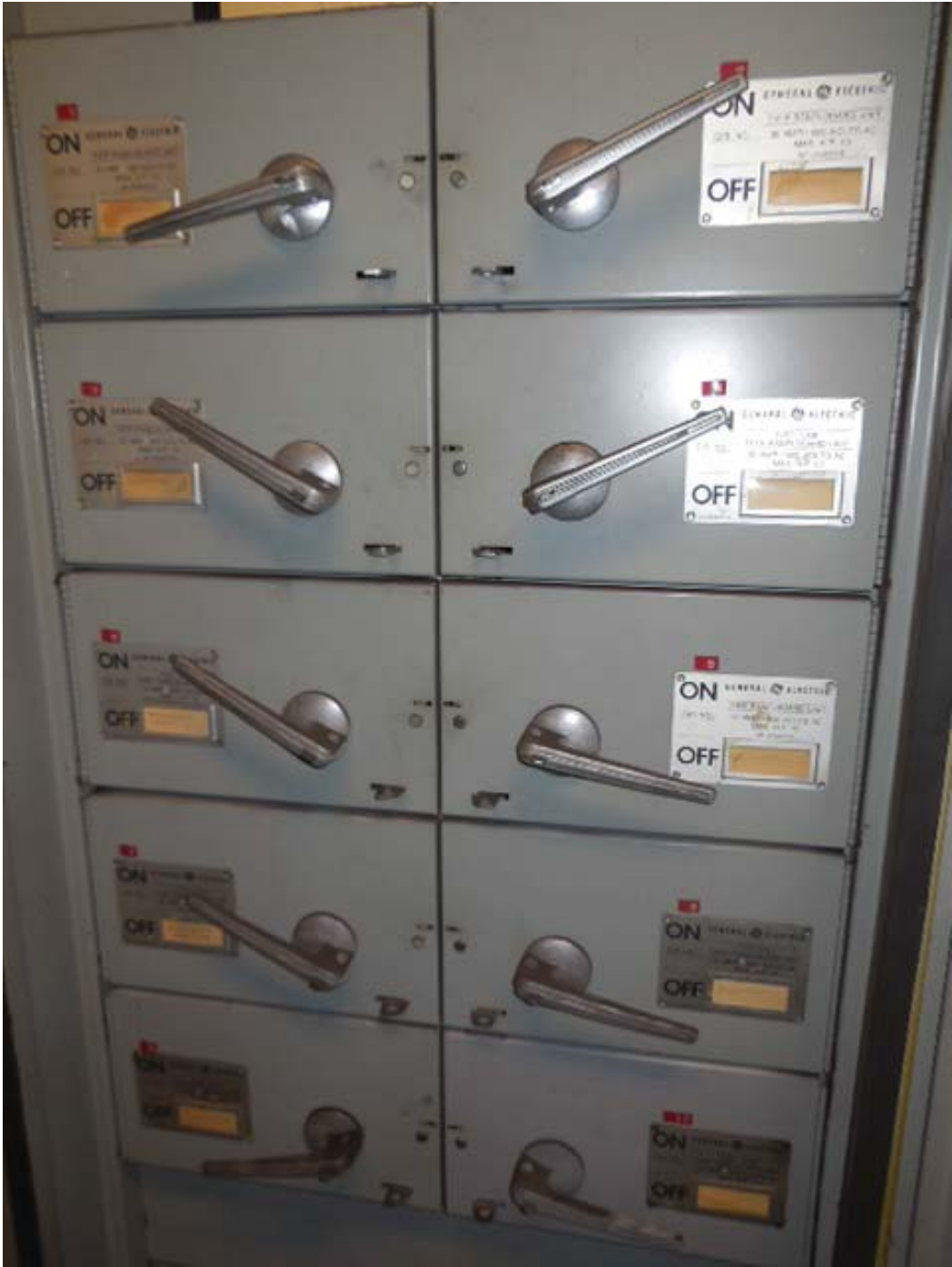
Picture 12: F06 Anacostia (South) – Panel SSE Emergency in room 302
