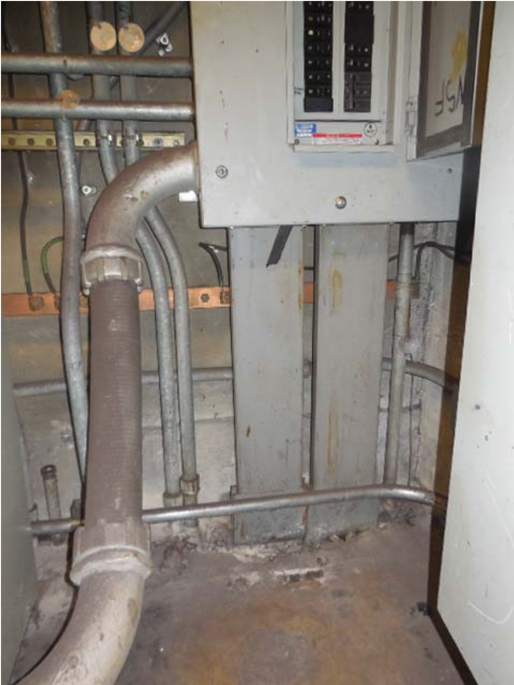
Picture 4: F06 Anacostia (North) – AFC Panel NSF in room 301, bottom ducts & conduit
