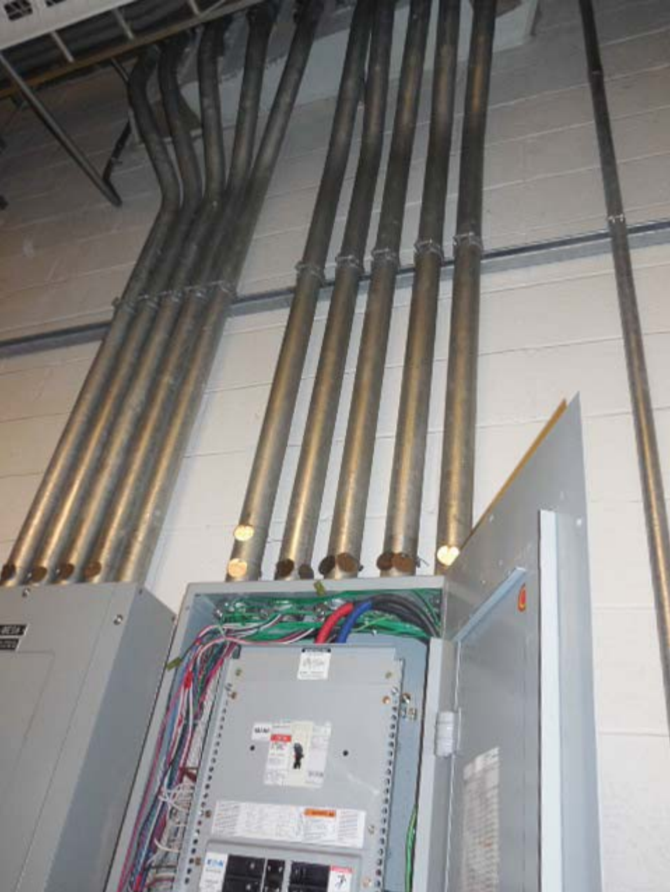
Photo #4: F05 Navy Yard (West) – Conduit risers from Panel WMESS in Room 401
