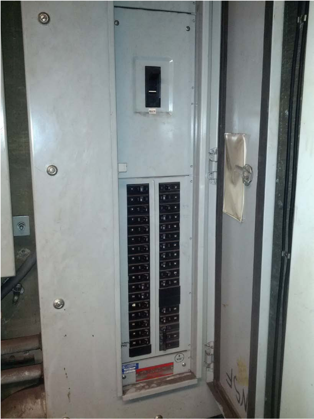
Picture 3: F06 Anacostia (North) – AFC Panel NSF in room 301
