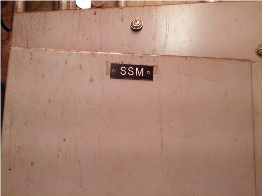
Picture 8: F06 Anacostia (South) – Panel SSM in room 302
