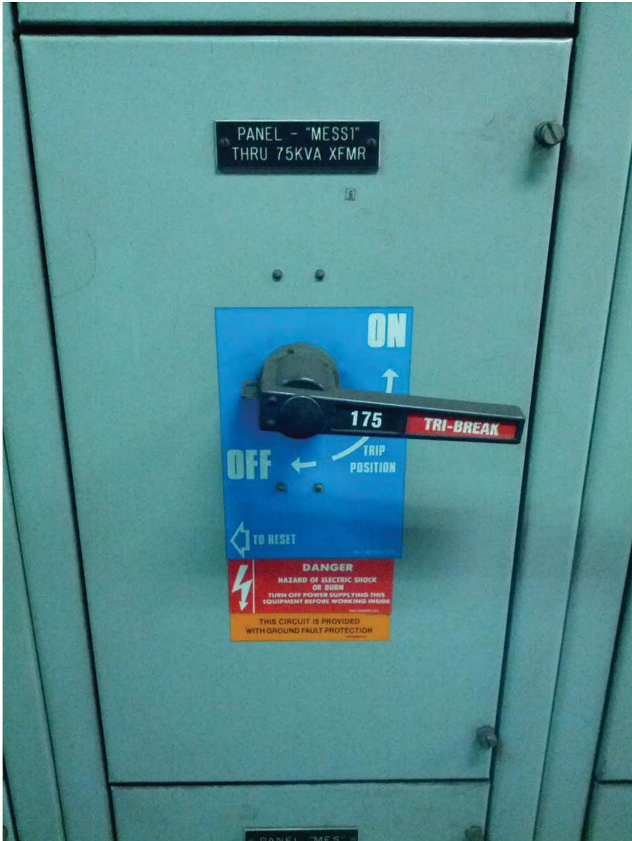
Picture 15: F04 Waterfront – WAC Essential Panel – XFMR Panel-MESS1 Circuit 6 in Room 203
