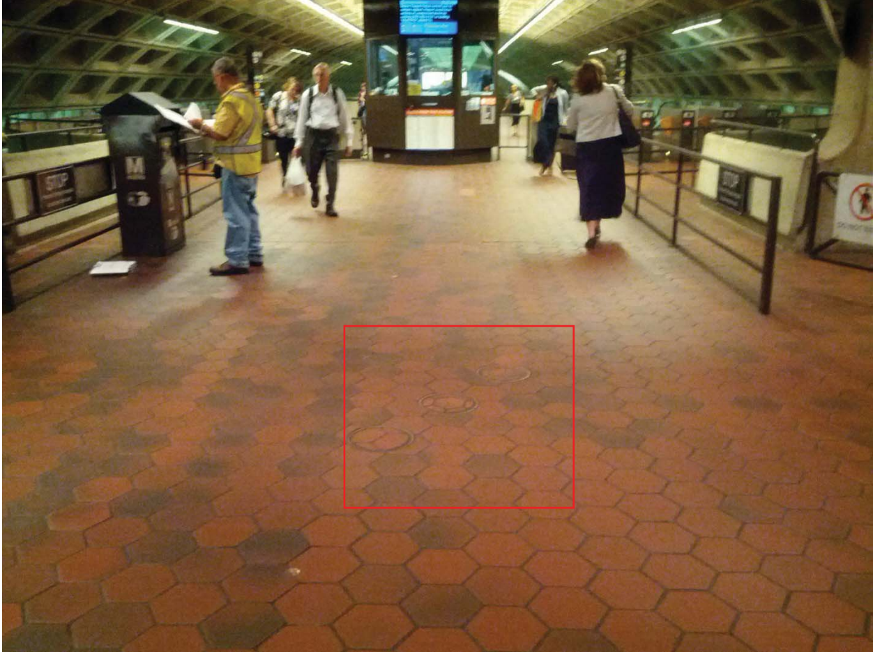
L'Enfant Plaza North Photo #17 – Handholes located on Mezzanine level about 35' feet from Kiosk
