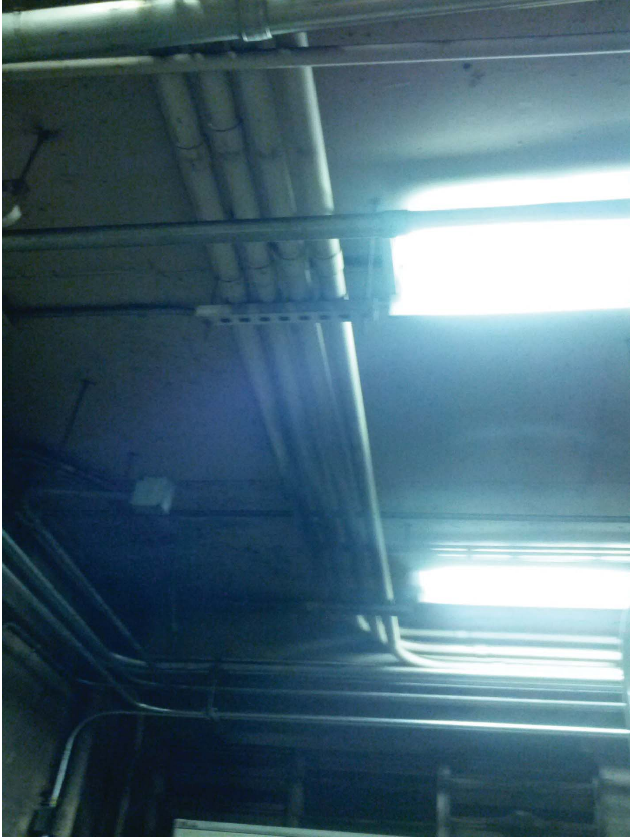
L'Enfant Plaza North Photo #7 –AFC Panel (NF) – Overhead Conduit Transition (Platform Level Rm. N104)
