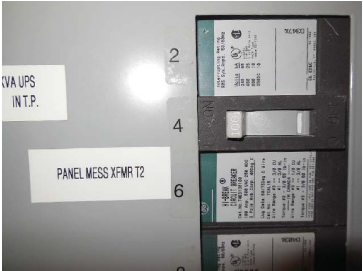
Picture 6: F08 Southern Ave – Generator Sub-panel 2 Circuits 2,4,6 in Room 223
